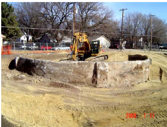
Filling the gas holder with clean fill. The bottom of the gas holder tank was broken to prevent water from continuing to collect in it.
