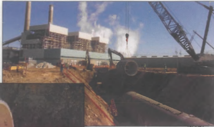
Construction on the circulating water line replacement on unit 3 at Jeffrey Energy Center.
