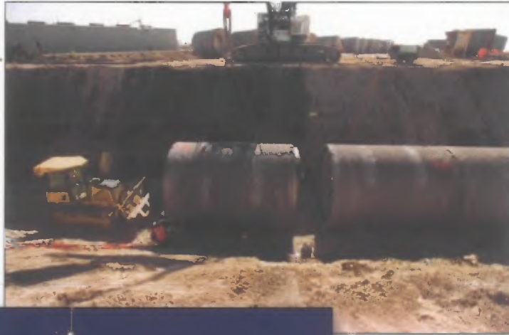
Construction on the circulating water line replacement on unit 3 at Jeffrey Energy Center.
