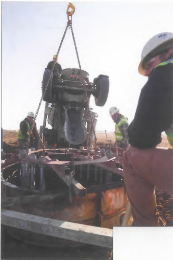
Contractors pour the concrete foundation for a steel pole for phase one of the 345 kV Wichita to Hutchinson to Salina line. Phase one extends from Wichita to Hutchinson. Phase two continues from Hutchinson to Salina.
