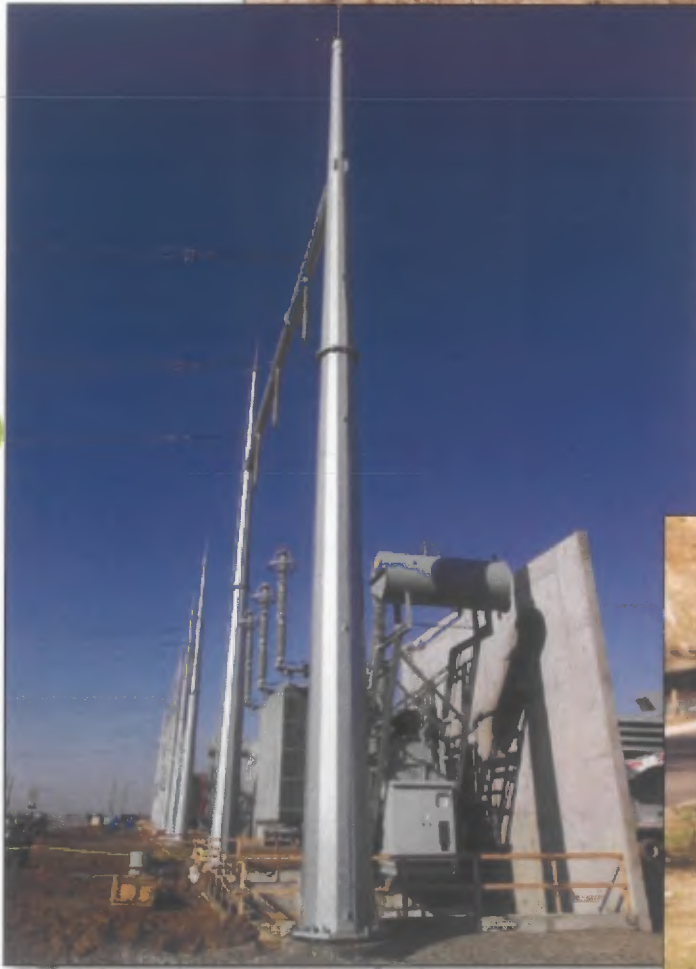
Transmission lines coming out of Emporia Energy Center.
