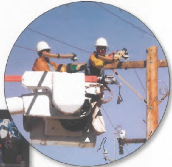
Ryan McCallister, apprentice lineman, and Robert Heath, journeyman lineman, install protective cover up on a line in preparation to provide service to a new commercial customer in DeSoto.
