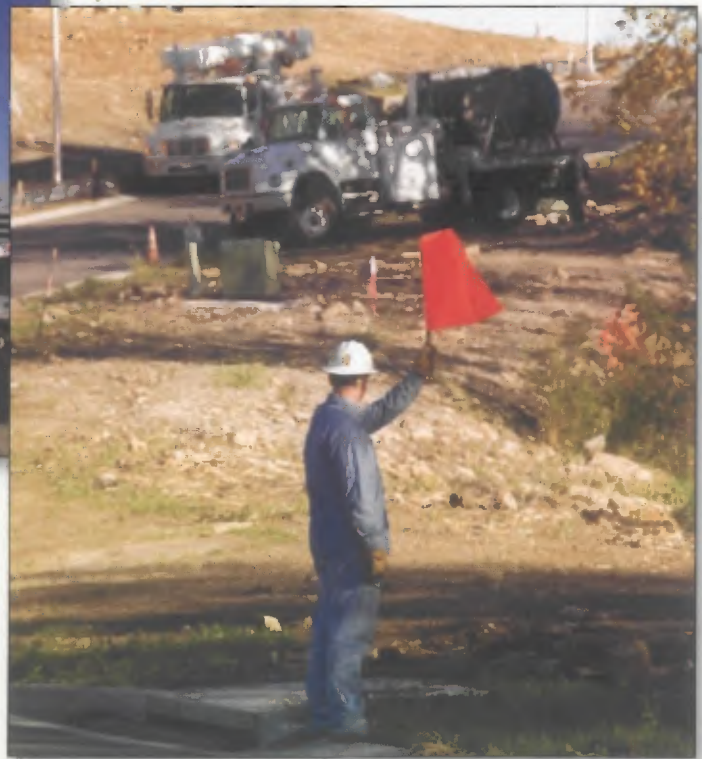
Todd Richardson, apprentice lineman, communicates with crew members as an underground cable is installed for a new residential development in Olathe.
