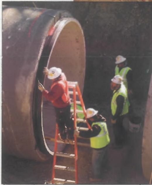
Crews prepare to seal a section of the new water line on unit 3.
