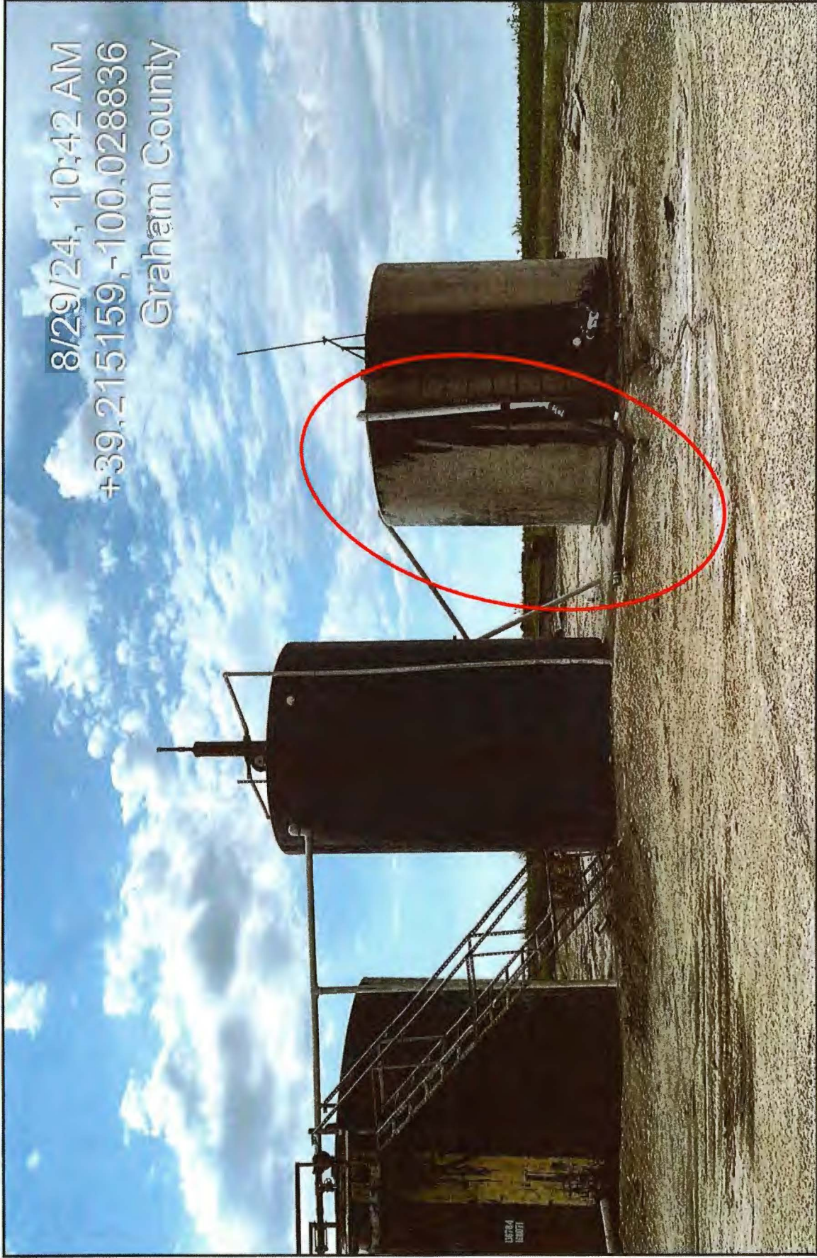
Above: The brine tank is equipped with a load line with a quick coupler on the end of the hose.
