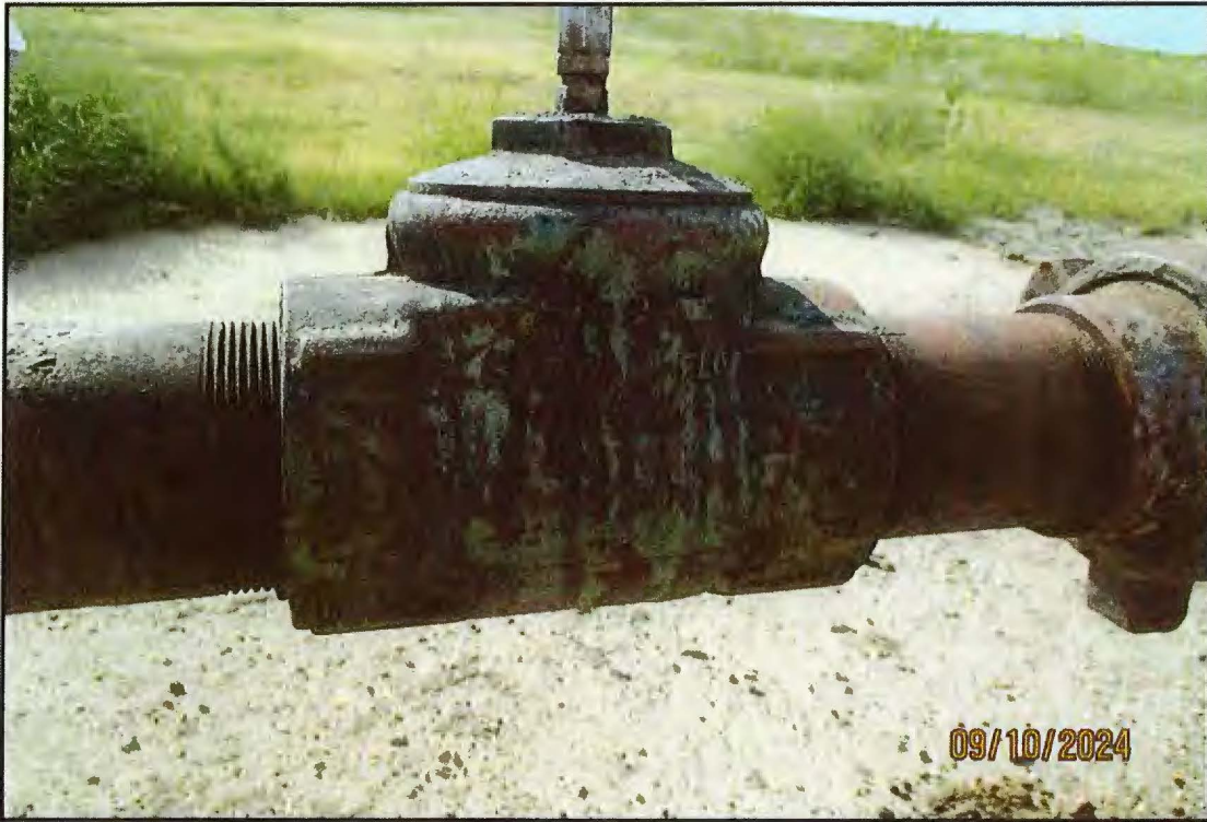
Above: View of the Breeden # 8 check valve located on the wellhead. The top of the check valve appears to have pipe wrench marks indicating that the flapper valve may have been accessed.
