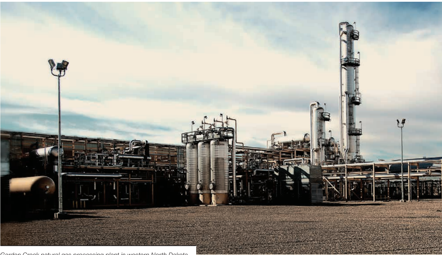
Garden Creek natural gas processing plant in western North Dakota.
