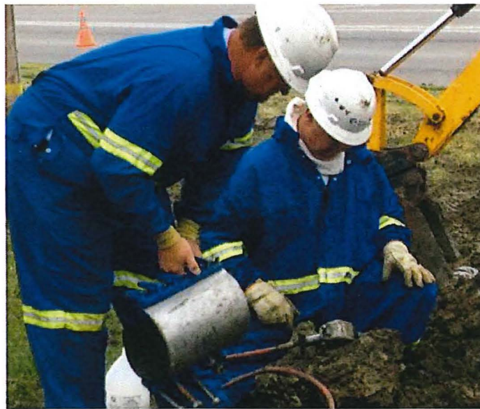
Repairing 8" main. Crew assistants with no fire protective hoods or air supply in potentially hazardous atmosphere
