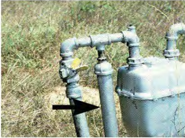
Figure 1: Wick-type odorizer near a gas meter.
