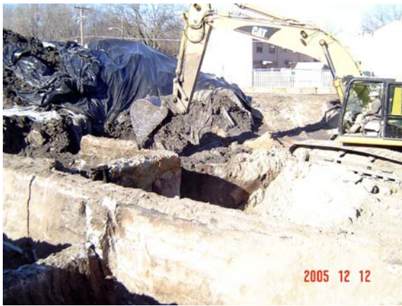
Excavation revealed underground foundations and structures. These were left in place when clean fill was installed.
