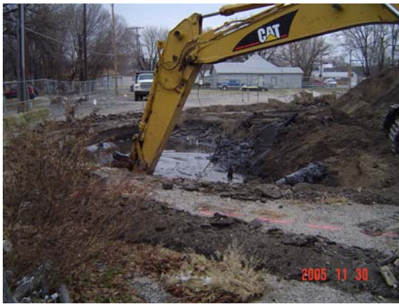
Removing the contents of the gas holder tank at the former manufactured gas plant in Manhattan. The contents are primarily water, woody debris, soil, and hard-parts refuse.
