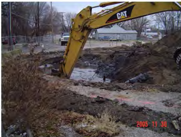
Removing the contents of the gas holder tank at the former manufactured gas plant in Manhattan. The contents are primarily water, woody debris, soil, and hard-parts refuse.
