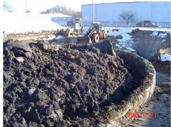
Excavated material from the site placed in the gas holder tank to soak up water contaminated with coal tar. The contaminated material was removed and properly disposed of at a hazardous waste disposal facility.
