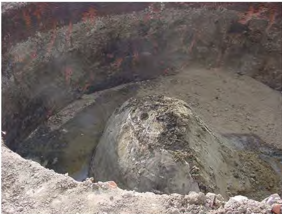
An excavated gas holder tank in Kansas City. In this picture is the “dumpling,” made of bedrock or concrete, usually left in the holder tank in order to support the gas holder framework and piping.
