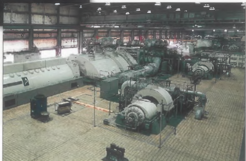
The turbine deck at Jeffrey Energy Center.
