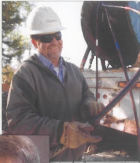
Craig Hansberry, Shawnee Division line foreman, prepares underground primary cable that will be used to service a new residential development.
