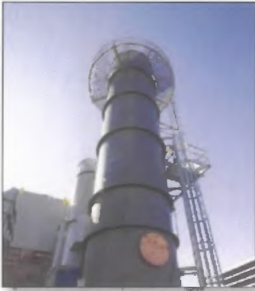
One of several stacks at the Emporia Energy Center.
