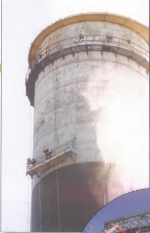
Crews clean one of the stacks at Jeffrey Energy Center as part of the scrubber retrofit.
